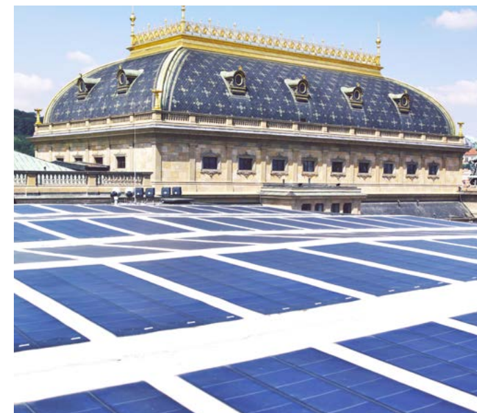
Even the historical center of Prague offers a number of opportunities for roof solar panels. The operating building of the National Theatre has a solar power plant installed since 2008, as part of the complex energy savings project. Today, the National Theatre saves about 50% of its original energy costs. PHOTO: NATIONAL THEATRE
